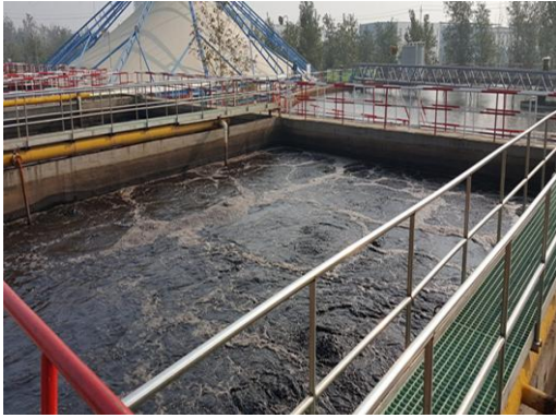
Fig.1: The sewage treatment project
